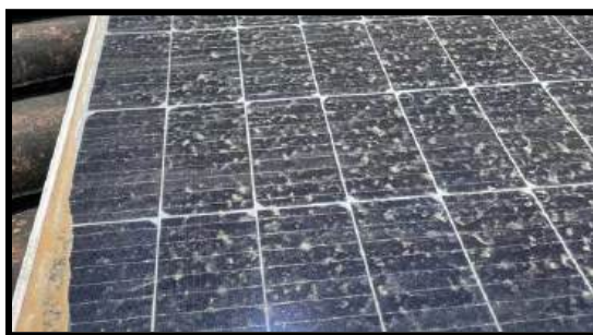
Above is a picture of a solar panel heavily affected by dust and dirt accumulation.
